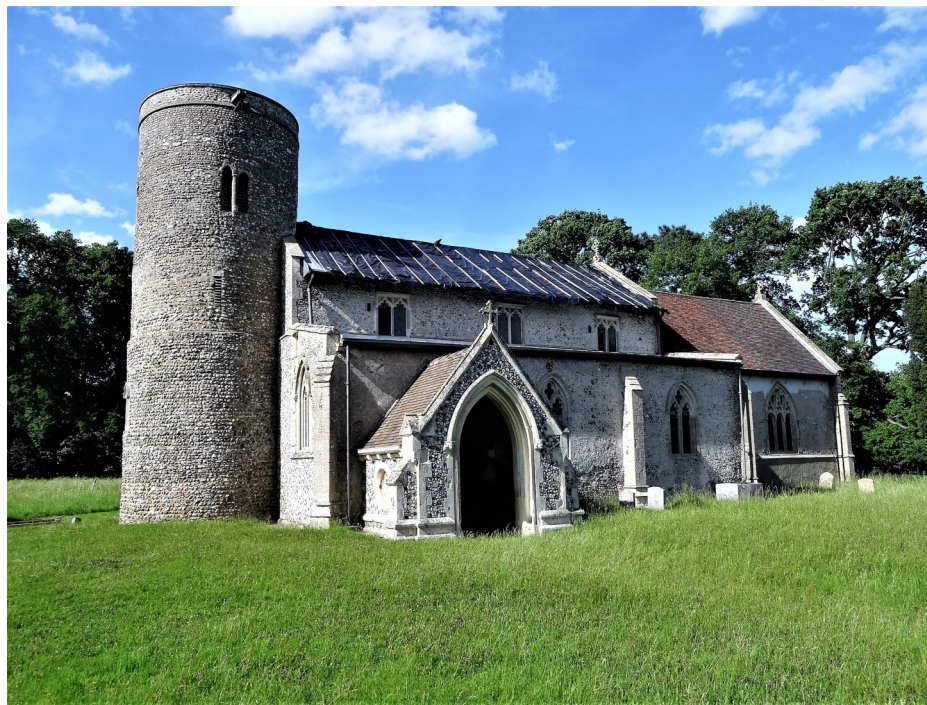
Merton St Peter with temporary plastic roof covering.
