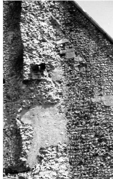
Pl.3 The breach in the tower south wall. Sloping dressed stones may indicate the original nave verge prior to the raising of the wall when the south aisle was built.
